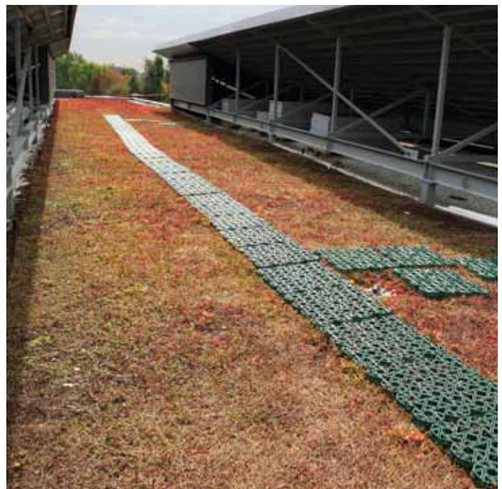
An example of temporary protection with grass pavers—sensitive plants need to be protected from rooftop maintenance traffic.
