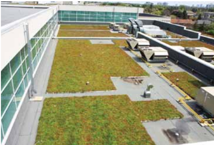
Splash pads and vegetation-free zones can be used to direct water from higher roof levels toward the drains. Space has also been left for gas pipes and rooftop units to allow for easier access and damage-free plants.
