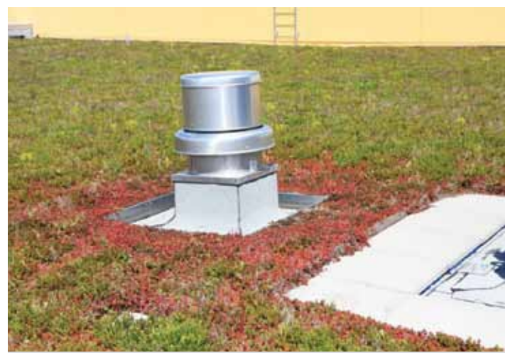
The design of a successful roof goes well beyond choosing plants and waterproofing. For example, direct exposure to air vents quickly dries out vegetation. Thoughtful placement of flora-free zones can help by making rooftop service work simple.
