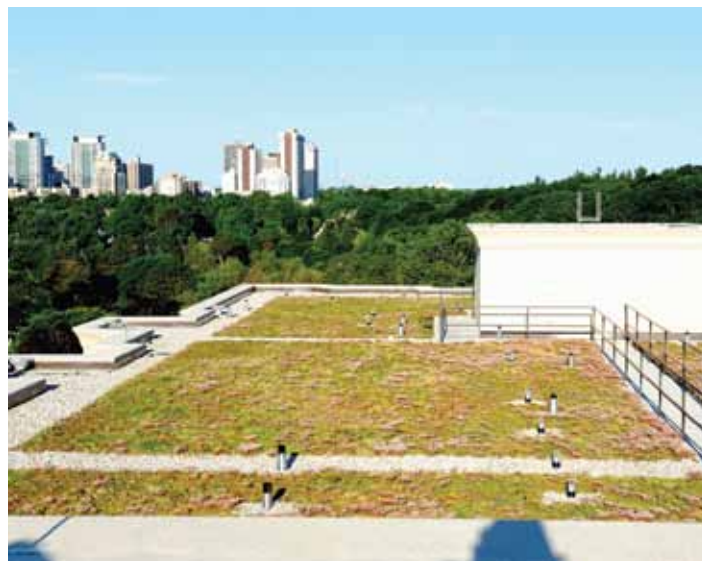
Vegetated roofs are essentially living building assemblies, with periodic needs for moisture and nutrients (as well as removal of unwanted plants). Ensuring regular maintenance needs to start with project design and be carried through the entire process—from design to building handover and beyond.
