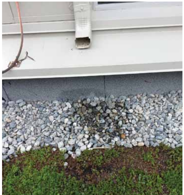
This close-up of a downspout shows the beginning of soil erosion. While it was beneficial to include the vegetation-free zone, it should have been larger.
