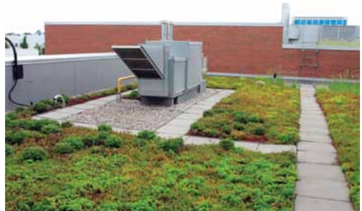
This photo shows a good example of how to create effective vegetation-free zones and access pathways to rooftop units and curbs.
